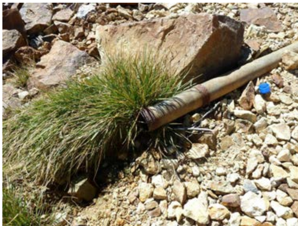
Photograph 12b: Pipe draining the upper Mary Ann Mine collapsed adit.
